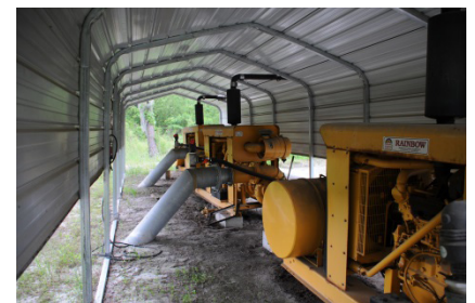
Figure 5. Diesel-powered prime movers for irrigation pumps.
